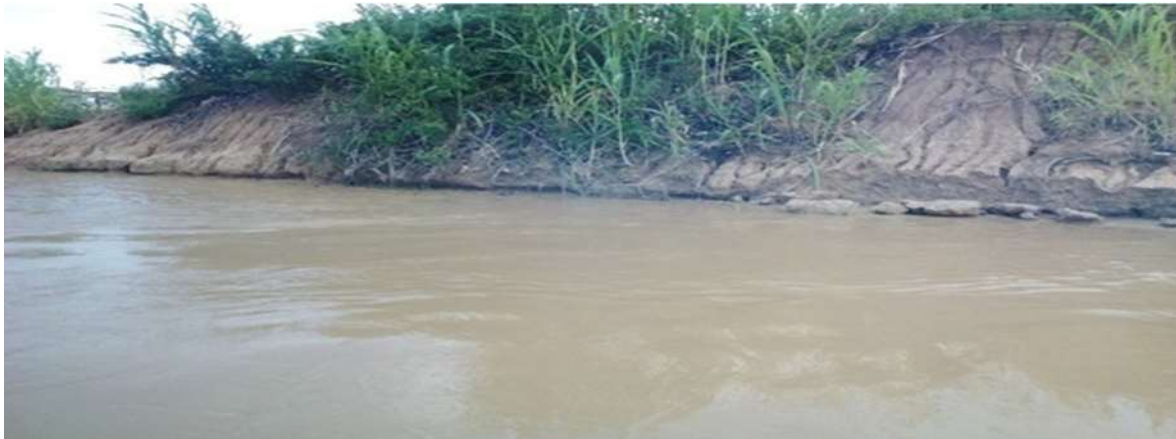
Figure 9: Two erosion processes occurring at the bank of the shoreline.
