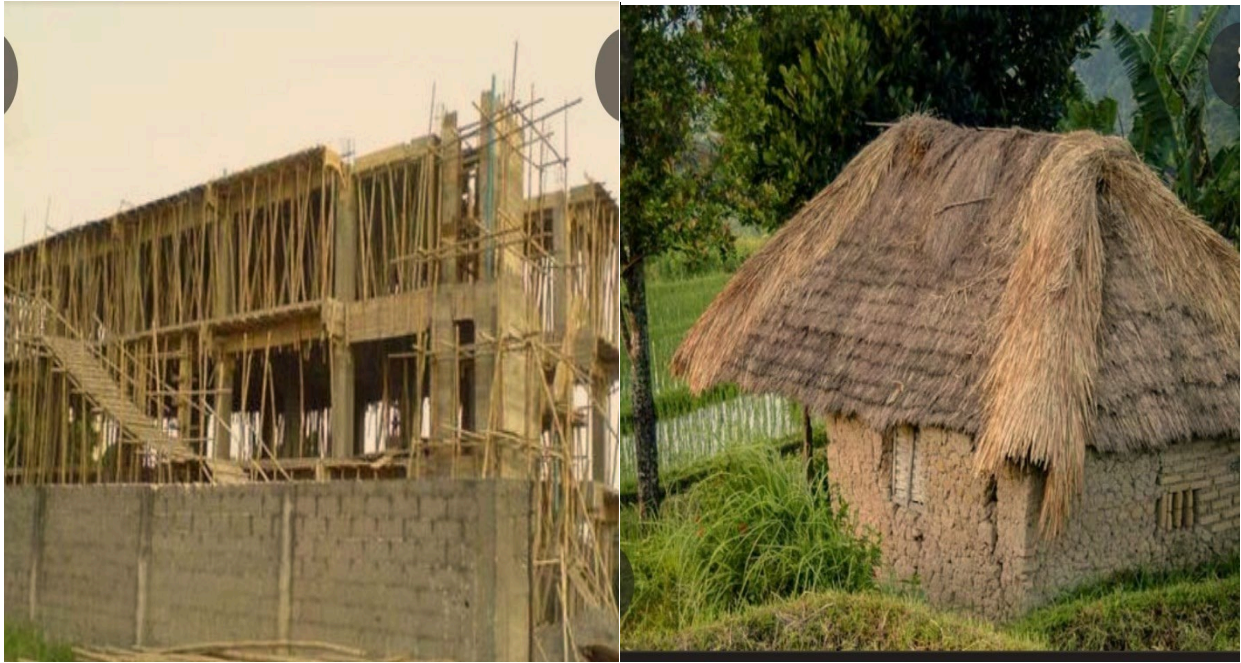
Figure 1: Bamboo used as scaffolding and a roofing element and structural base in mud house.
